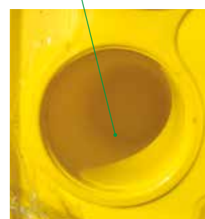
Clean water tank
